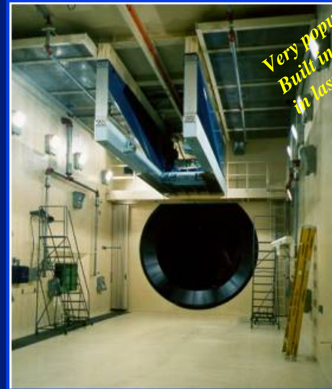
7M x 7M test facility for regional Jet
